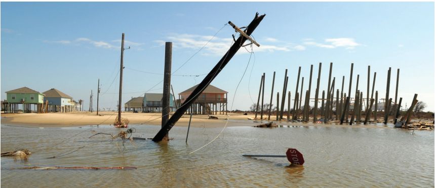
Bolivar Peninsula, TX, September 20, 2008: Damaged houses, debris and downed power lines resulting from Hurricane Ike. Photo by Jocelyn Augustino, FEMA.
